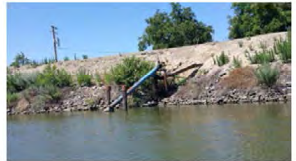
Closer view of the erosion.
