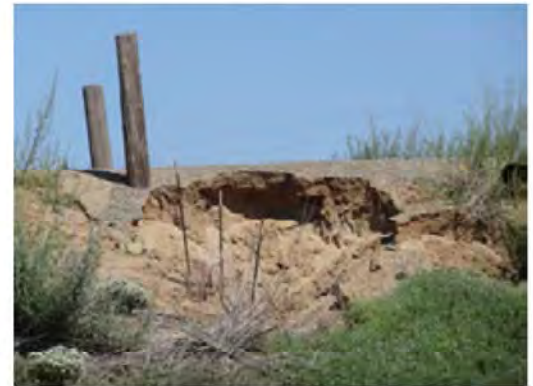
Close view of the erosion.
