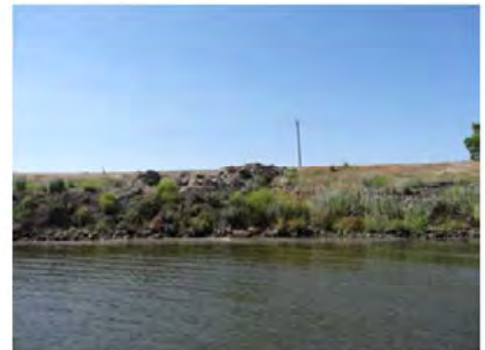
Front view of the erosion.
