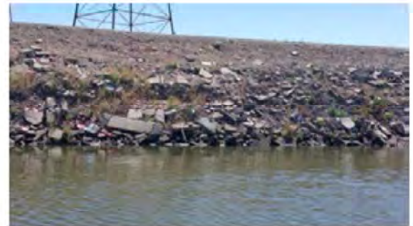
Close view of the erosion. The slope protection is poor.
