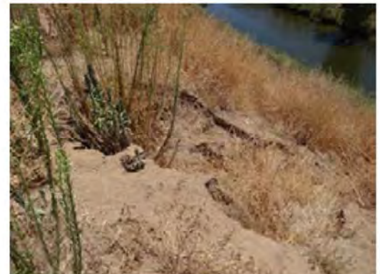
Close view of the erosion.
