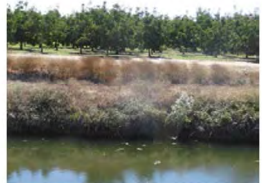
Front view of the erosion.
