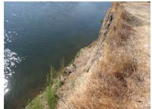
Direct view of the erosion.
