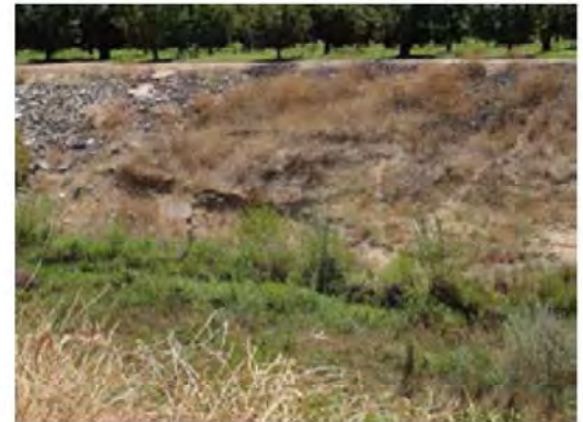
Close view of the erosion.
