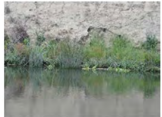
Close view of the erosion.
