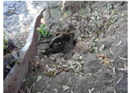
Close view of the erosion.
