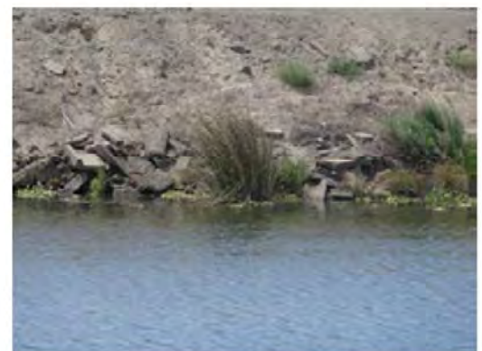
Close view of the erosion.
