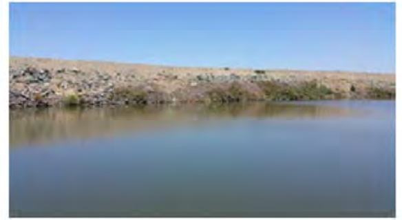
Front view of the erosion site.
