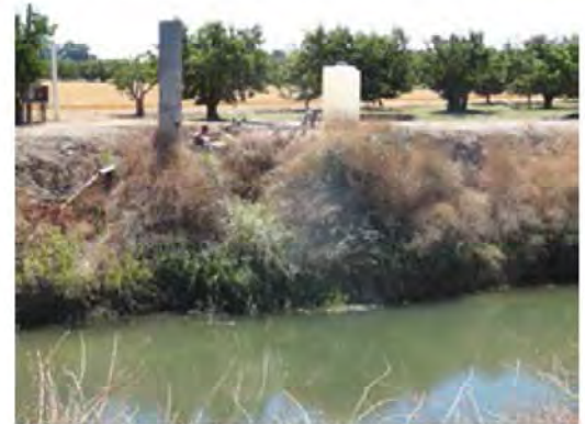
Front view of the erosion.
