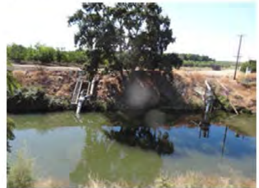
Front view of the erosion.
