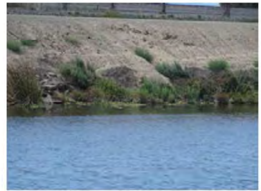
Front view of the erosion site. Note the vegetation at the levee toe and on the lower slope.
