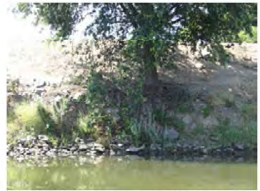
Front view of the erosion site. Note the large tree above the erosion.
