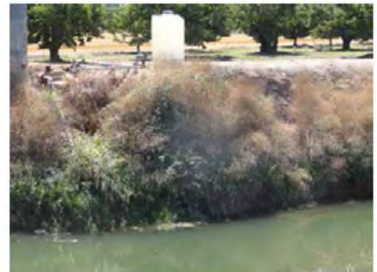
Closer view of the erosion.
