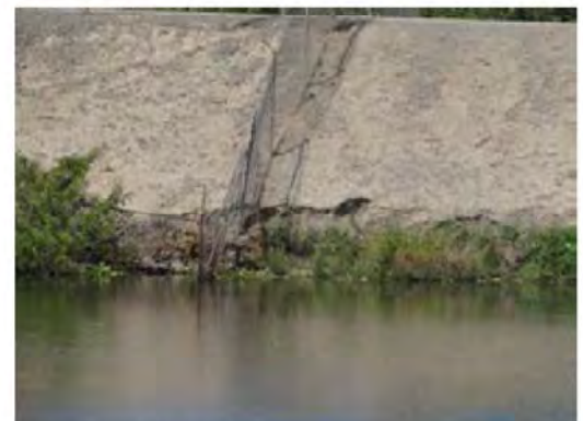
Front view of the erosion.
