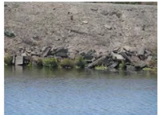
Close view of the erosion.
