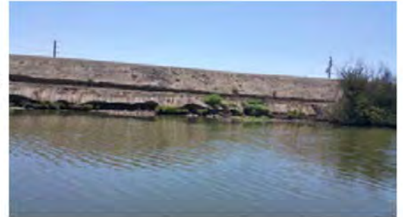
Front view of the erosion.
