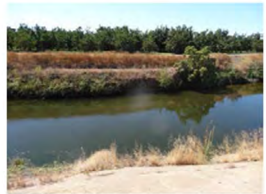
Front view of the erosion site.
