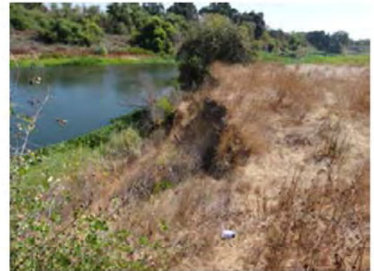
Downstream view of the erosion.
