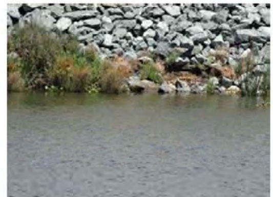
Close view of the repaired erosion site. Note the minor erosion at the water edge.
