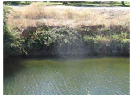
Closer view of the erosion.
