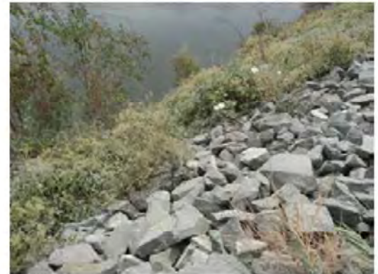
The erosion is not visible from the levee top. The levee slope is protected by riprap rocks.
