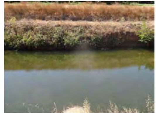
Close view of the erosion.
