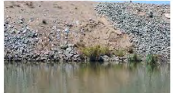
Front view of the erosion.
