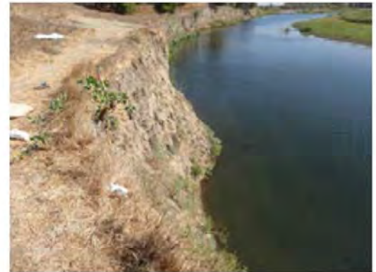
Close view of the erosion.
