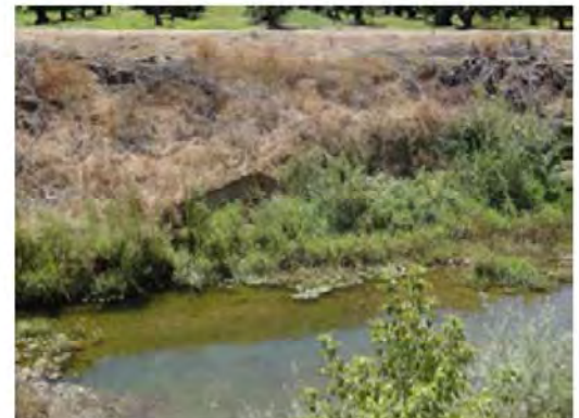
Close view of the erosion.
