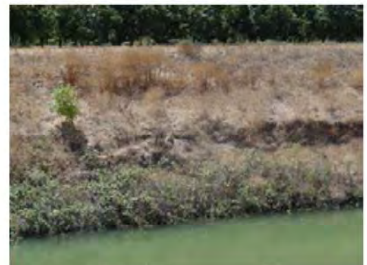
Front view of the erosion.
