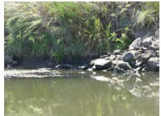
Close view of the erosion.
