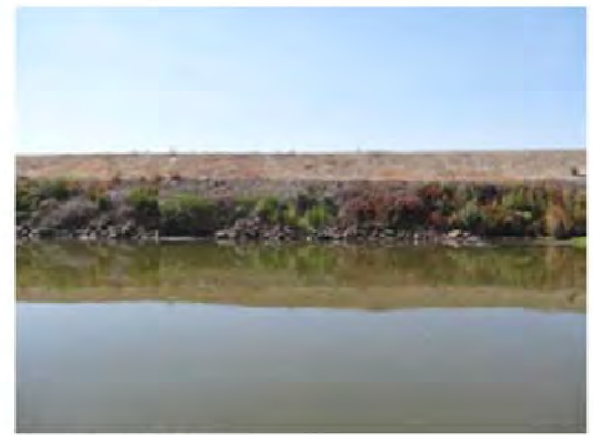
Front view of the erosion.
