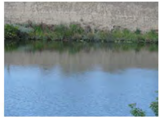
Close view of the erosion.
