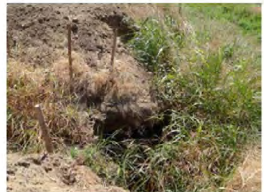
Close view of the minor erosion at the lower bank slope.
