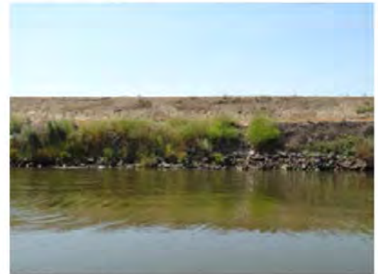
Front view of the erosion.
