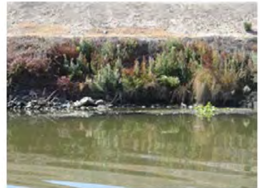
Front view of the erosion.
