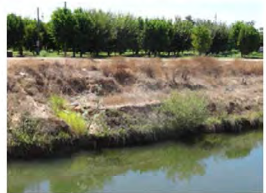
Closer view of the erosion.
