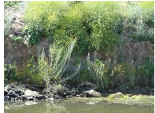
Close view of the pocket erosion.
