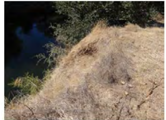
Close view of the erosion. Note the dense vegetation and tree on site.
