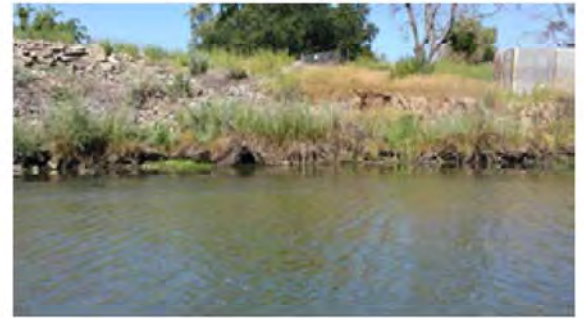
Front view of the erosion.
