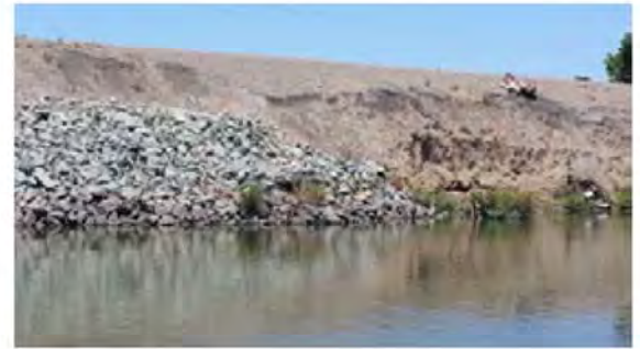
Front view of the erosion.
