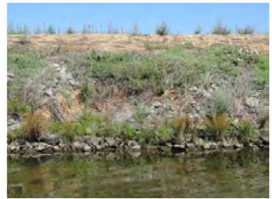
Front view of pocket erosion. Note the vegetation and riprap at the site.
