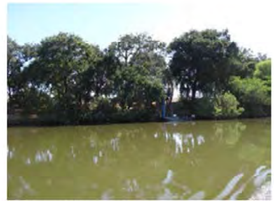
Front view of the erosion site. View is partially blocked by the pump structure and vegetation.
