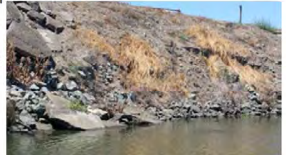
Close view of the erosion.
