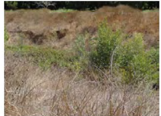
Closer view of the erosion.
