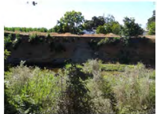
Close view of the erosion. Signs of new erosion along the site.
