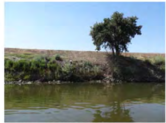
View of the pocket erosion and the tree.
