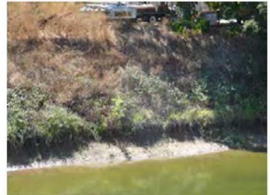
Close view of the erosion.
