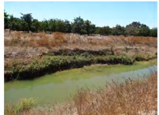
Front view of the erosion.
