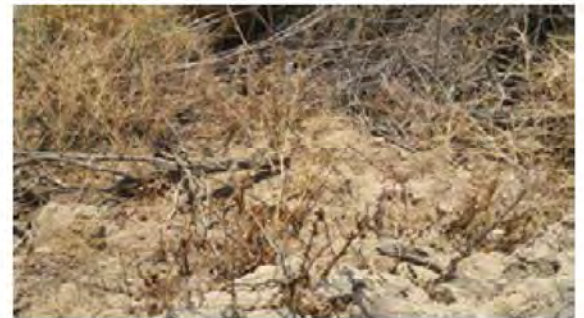
Direct view of the erosion. Note dense vegetation at the site.
