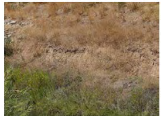
Close view of the erosion.
