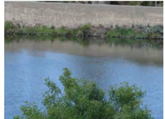
Close view of the erosion.
