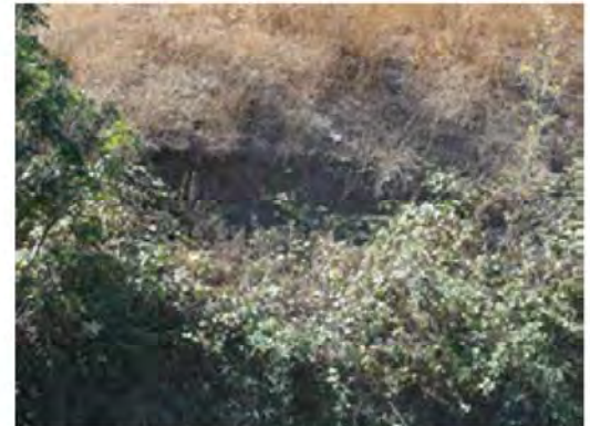
Close view of the pocket erosion.
