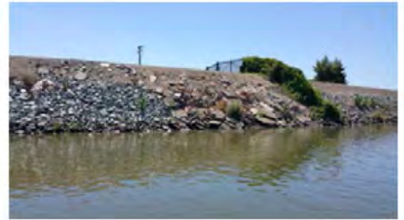
Front view of the erosion site. Note the concrete blocks and vegetation.
