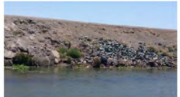
Close view of the erosion. The upstream end of the site is protected by riprap revetment.
