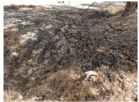
View of the erosion site from the levee crest.
