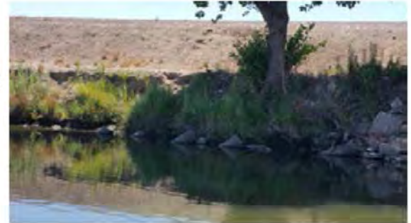
Close view of the erosion.
