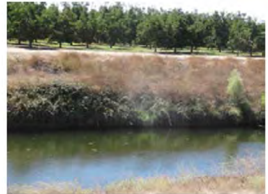
Close view of the erosion.
