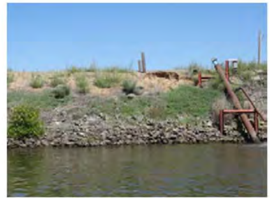
Front view of the erosion site.
