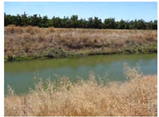
Front view of the erosion.
