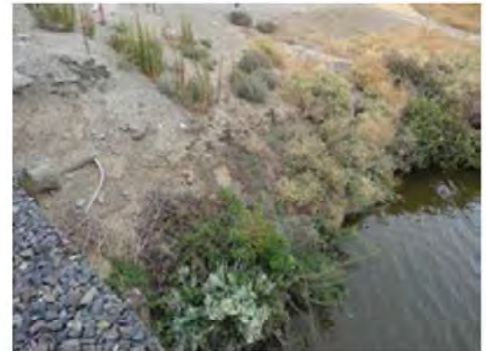
Looking down at the erosion downstream of the Railroad bridge.
