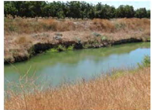
Close view of the erosion.
