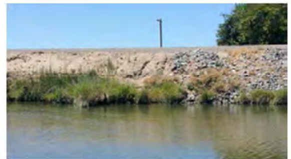
Close view of the upstream side of the erosion.
