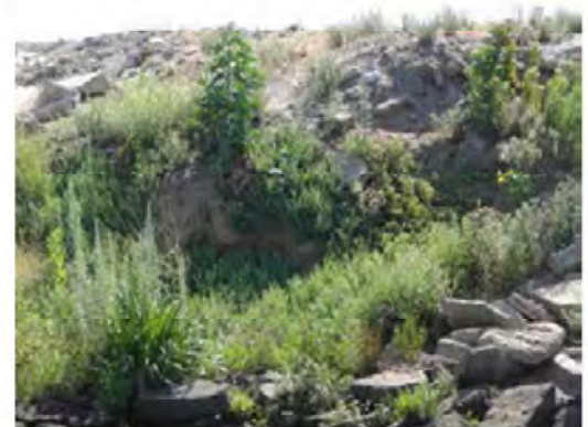
Front view of the site. Rip rap no longer adequately protecting levee slope.
