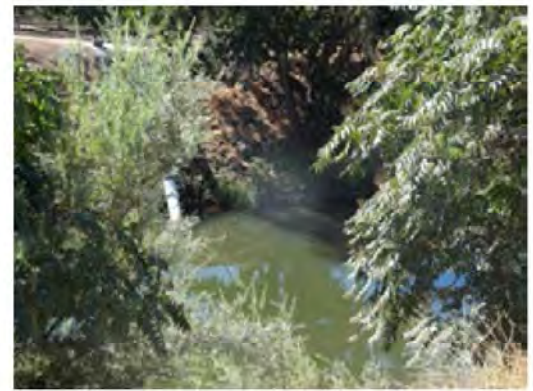
Front view of the erosion. The erosion is next to a tree at the levee toe.
