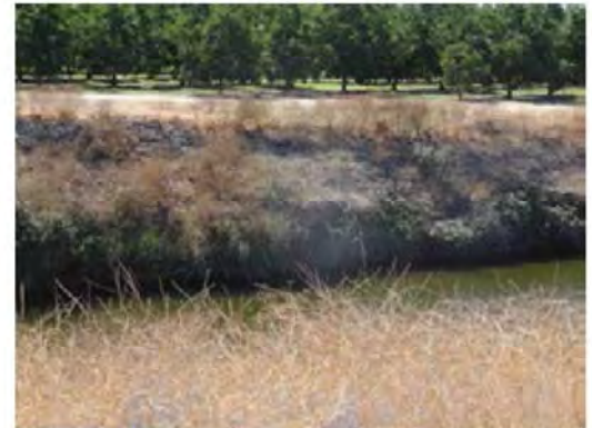
Front view of the erosion.
