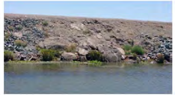
Front view of the erosion.
