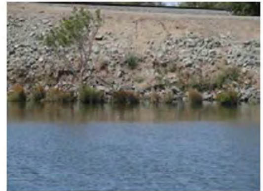
Close view of the erosion.
