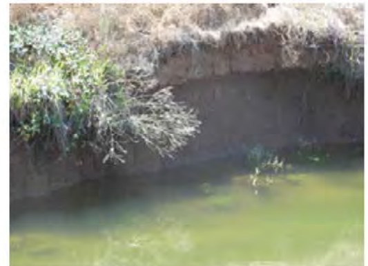
Close view of the erosion.
