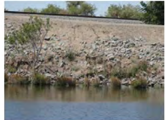
Close view of the erosion.
