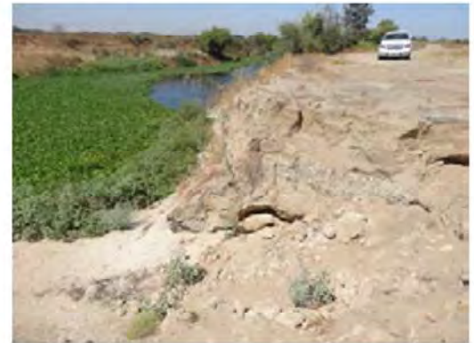
Looking upstream. Note the pocket erosion.
