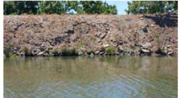
Close view of the erosion.
