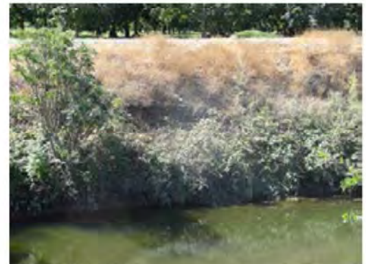
Close view of the erosion.
