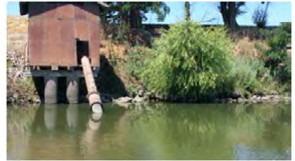
Front view of the erosion.
