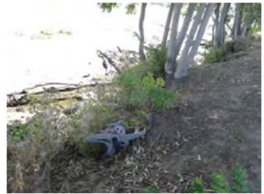
Front view of the site where undermining has occurred.
