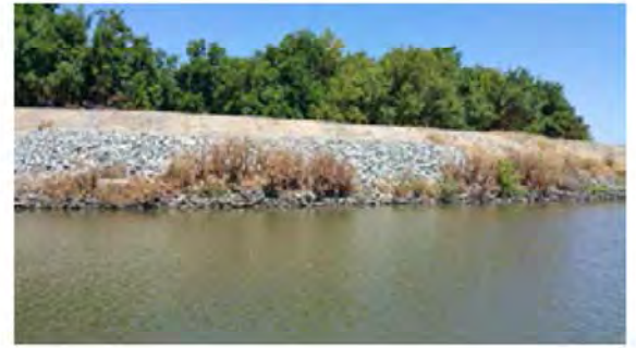
View of the repaired site. Note the new erosion at the levee toe.
