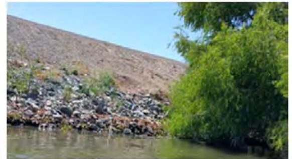
Close view of the repaired erosion site. Note the tree near the site.
