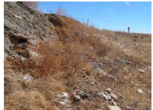
Looking downstream at the erosion site.
