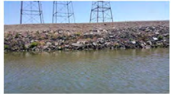
Front view of the erosion.
