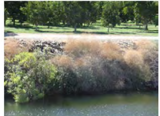
Close view of the erosion.
