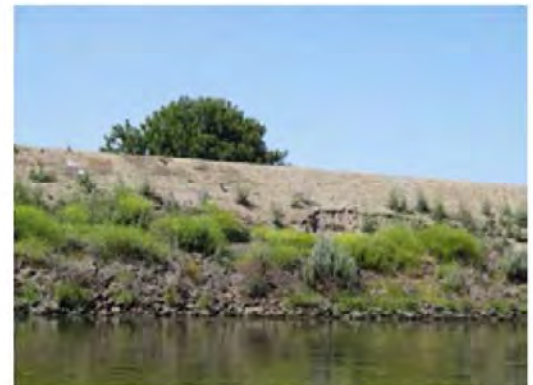
Front view of the site. Note the crack along the middle of the slope.
