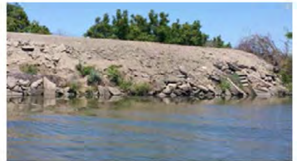
Front view of the site. Note the loosely placed concrete blocks.
