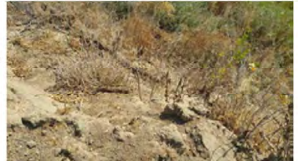
Close view of the erosion.
