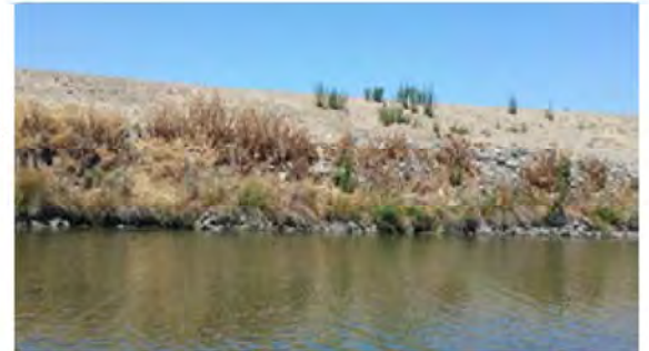
Close view of the erosion.
