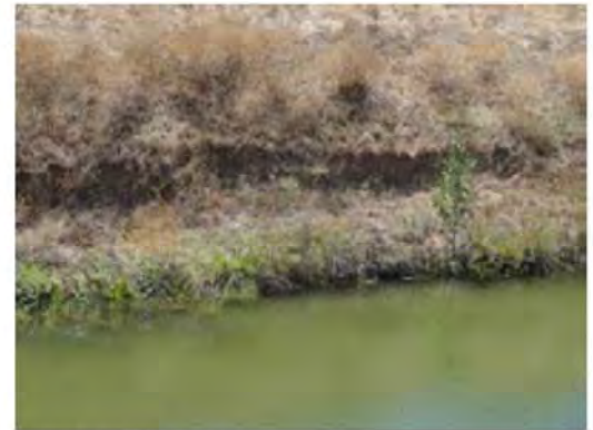
Close view of the erosion.
