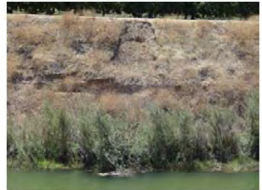
Close view of the erosion.
