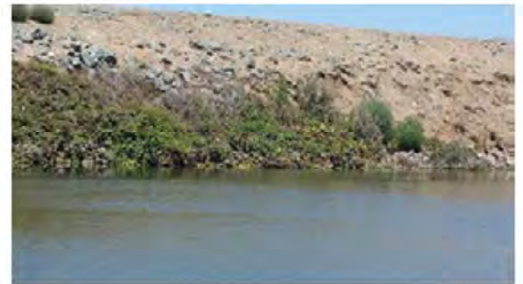
Close view of the erosion. Note the vegetation at the site.
