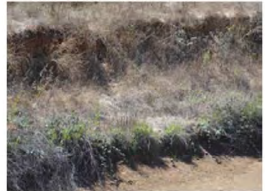
Closer view of the erosion.
