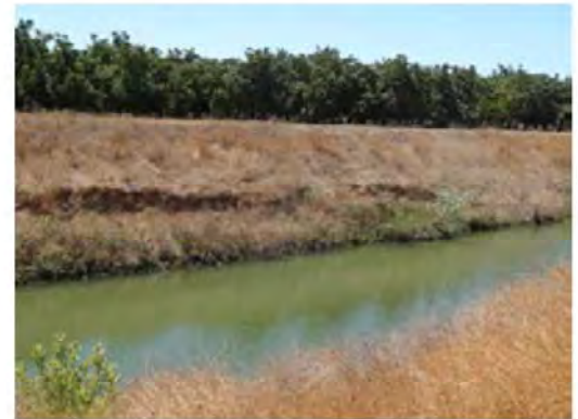
Close view of the erosion.
