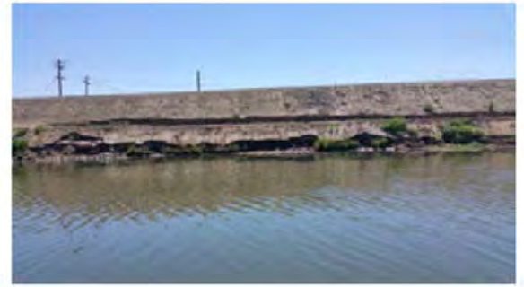
Front view of the erosion site. Note the new cut at the middle levee slope.
