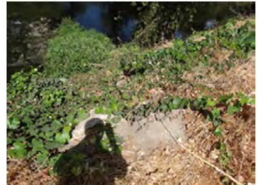
View of the current condition of the bank slope just above the irrigation outlet.
