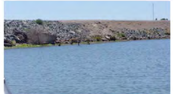
Close view of the erosion. Note the protection on the lower levee slope.
