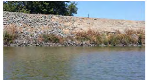
Front view of the erosion.
