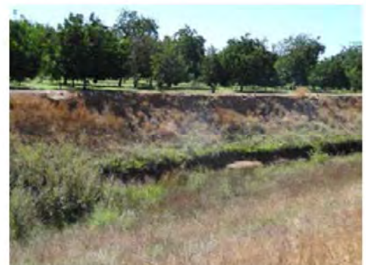
Close view of the erosion.
