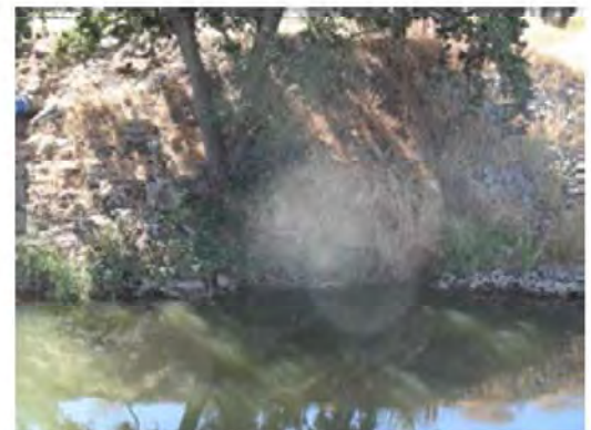
Closer view of the erosion.
