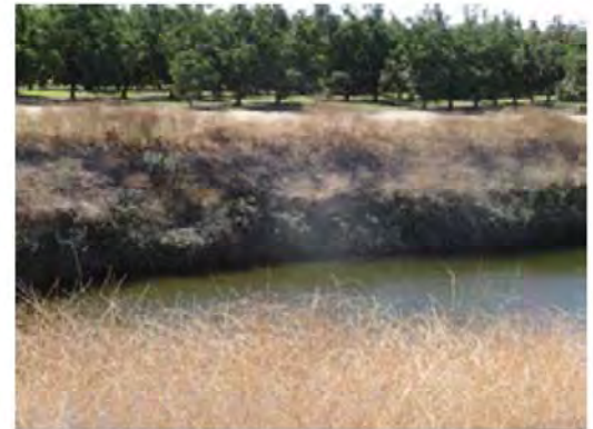
Front view of the erosion.
