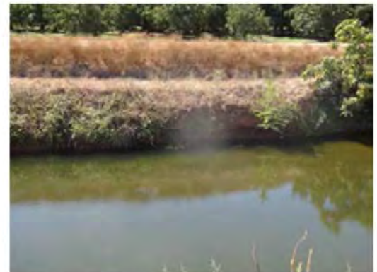
Close view of the erosion.
