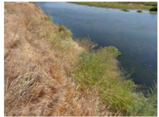
View of the downstream end of the erosion.
