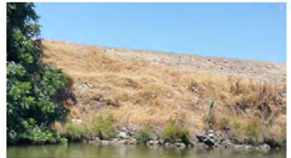
Closer view of the erosion.
