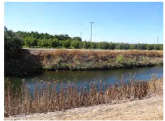
Front view of the erosion.
