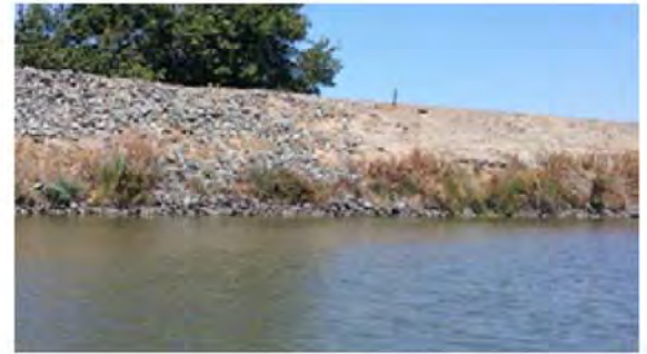
View from upstream of the erosion.
