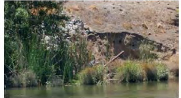
A close view of the erosion.
