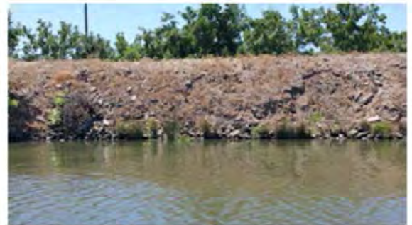
Close view of the erosion.
