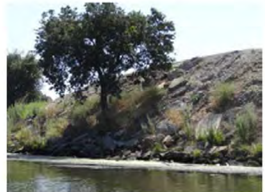
Front view of the site. Note existing broken concrete on the upper slope as well as on the lower slope and at the toe.
