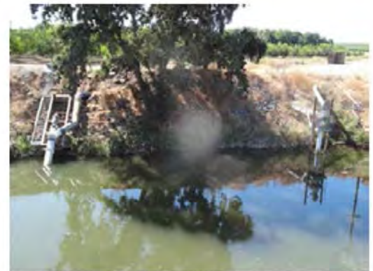
Front view of the erosion and broken concrete protection on the levee slope.
