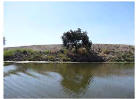
Front view of the erosion site.
