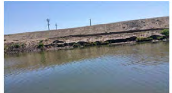
Front view of the erosion.
