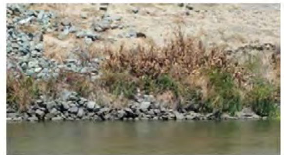
Close view of the erosion. Note river rocks and vegetation at the levee toe.
