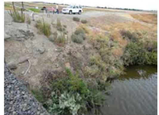
Close view of the erosion downstream of the RR bridge.
