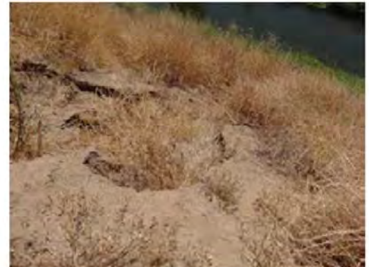
Close view of the erosion.
