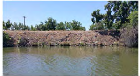
Front view of the erosion.
