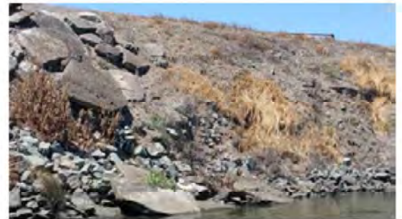
Close view of the erosion.
