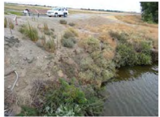
Direct view of the erosion upstream of Railroad bridge.
