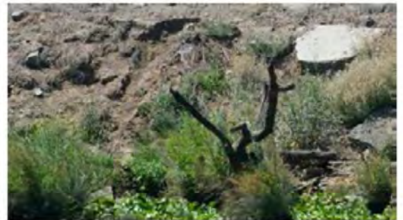
Close view of the pocket erosion. Note the vegetation at the site.
