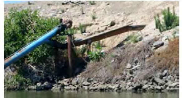
Close view of the erosion and the pipe.
