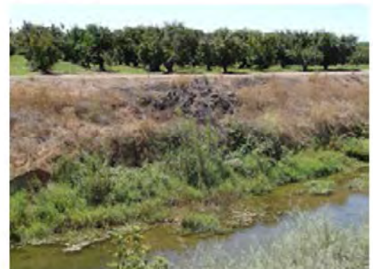
Close view of the erosion.
