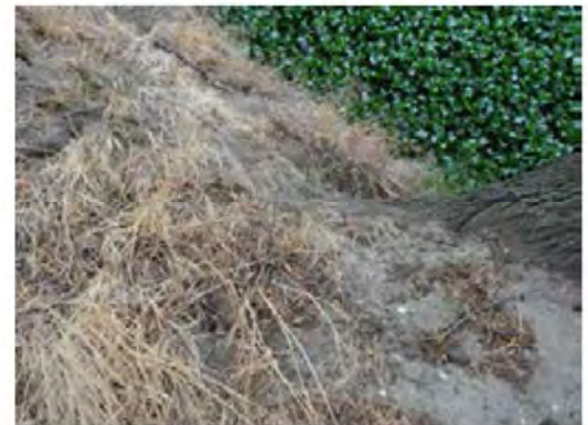
Direct view of the erosion near a tree.
