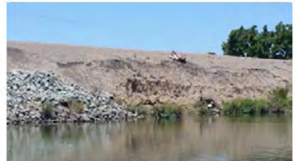
Front view of the erosion.
