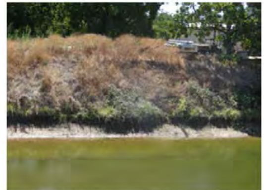
Close view of the erosion.
