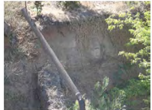
Close view of the erosion.
