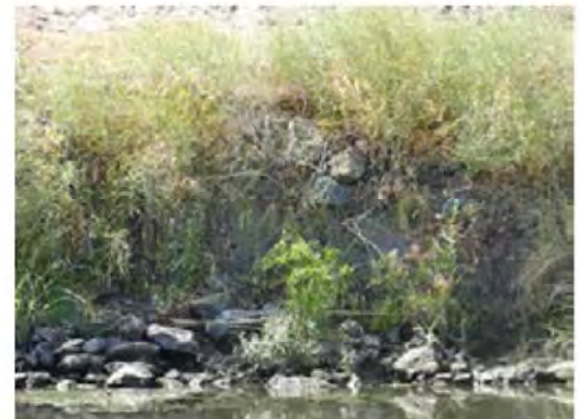
Close view of the erosion.
