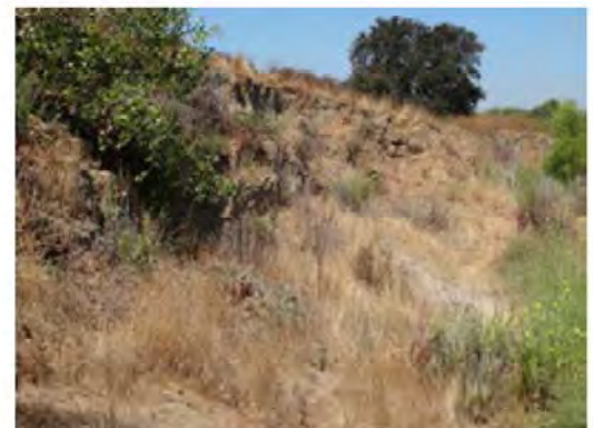
Close view of the erosion. Levee crest is approximately 8 feet above the erosion.
