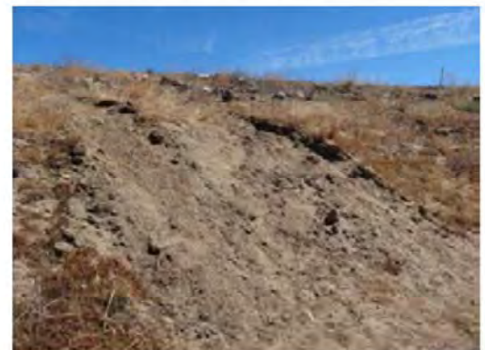
Direct view of the levee slope. Note the loose soil possibly caused by runoff.
