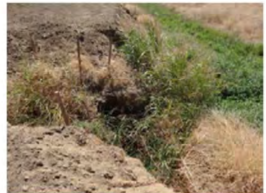
The erosion site has been repaired but a minor erosion at the lower bank slope is still visible.
