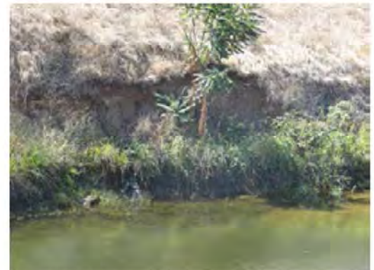
Close view of the scarp erosion. Note the small tree at the erosion site.
