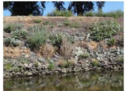
Close view of the erosion.
