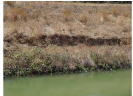
Close view of the erosion.
