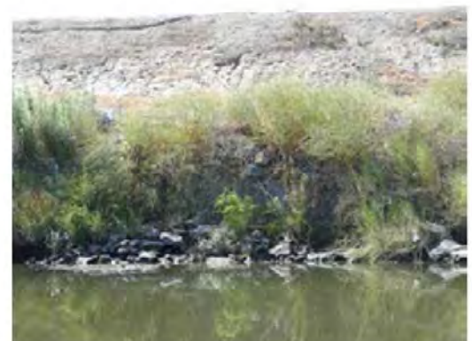
Close view of the erosion.
