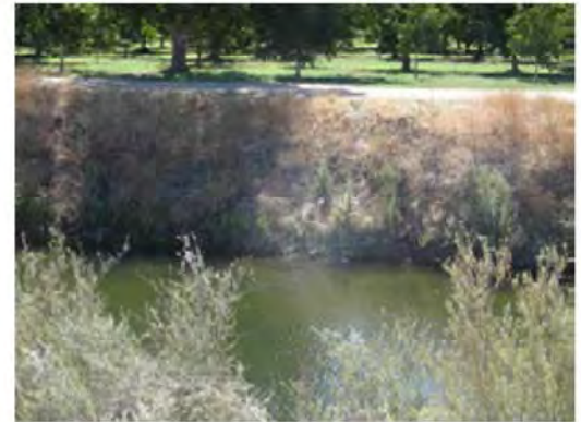
Close view of the erosion.
