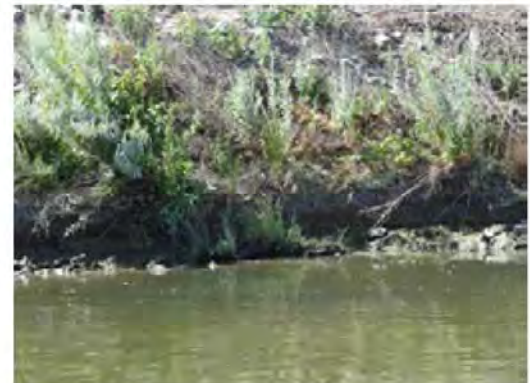
Front view of the existing erosion at the toe.
