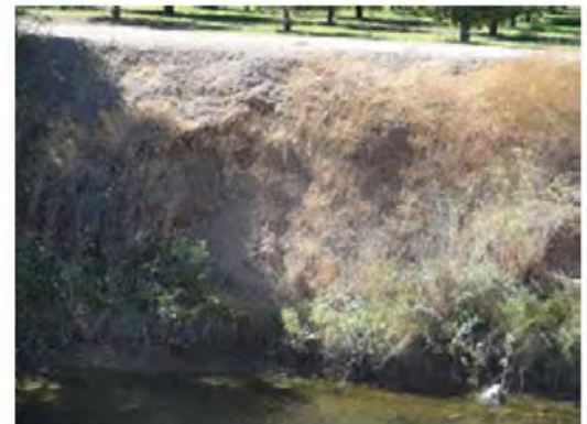
Close view of the erosion.
