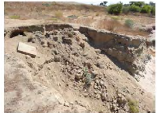
Close view of the pocket erosion.
