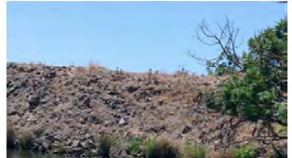
Close view of the erosion.
