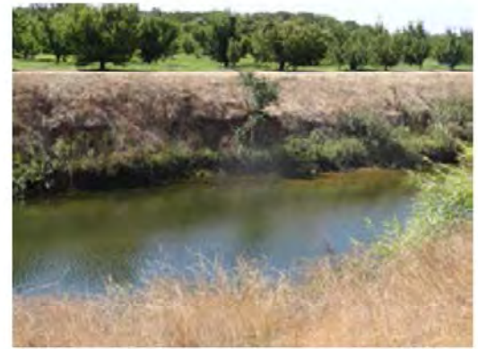
Front view of the erosion.
