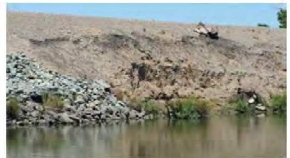
Front view of the erosion.
