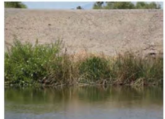
Front view of the erosion.
