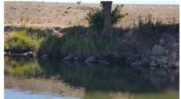
Close view of the erosion.
