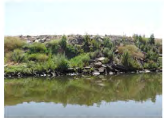
Front view of the site. Previously placed rip rap slipped, exposing the underlying soils and creating a pocket.
