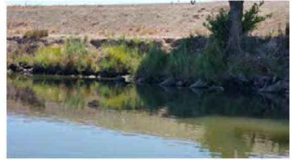
Front view of the erosion. Note the tree and the irrigation pipe.
