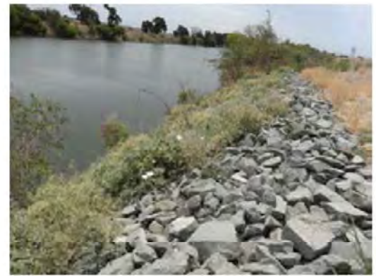
View of the erosion from the survey boat. The dense vegetation on the site blocks the view of the erosion.
