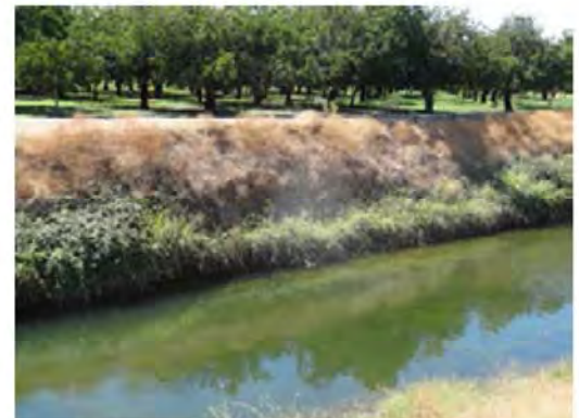
Close view of the erosion. Note the dense vegetation.
