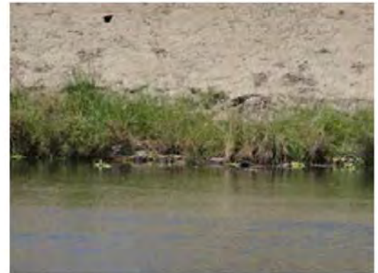
Front view of the erosion site. Vegetation is visible.
