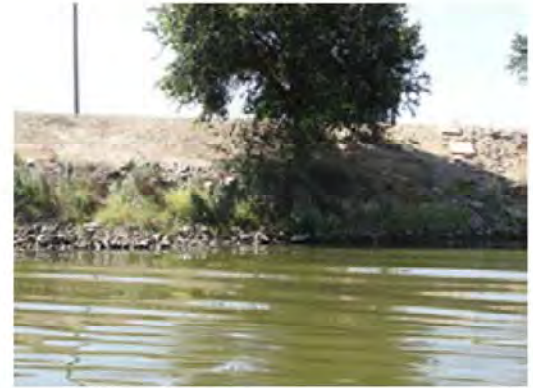
Close view of the erosion.
