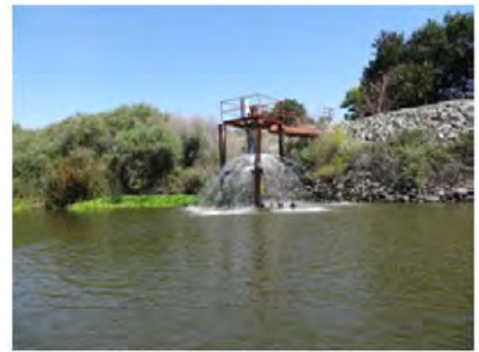
Front view of the site. The irrigation pipe is functioning and leaking water at the site.
