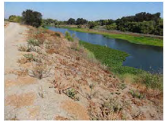
Upstream view of the erosion.
