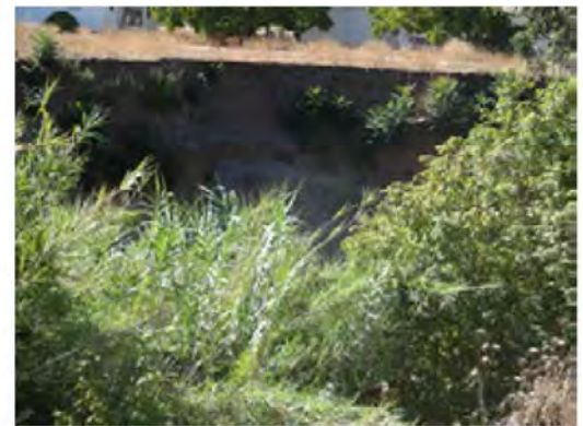
Close view of the erosion.
