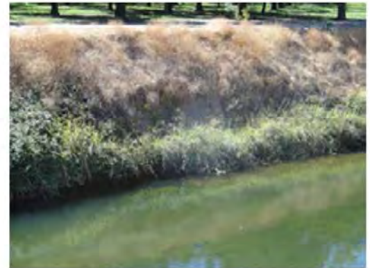
Close view of the erosion.
