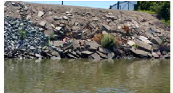
Close view of the erosion.
