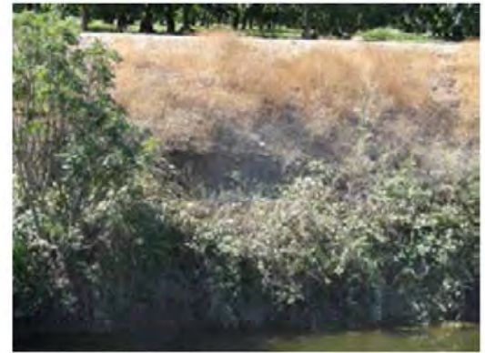
Front view of the pocket erosion.
