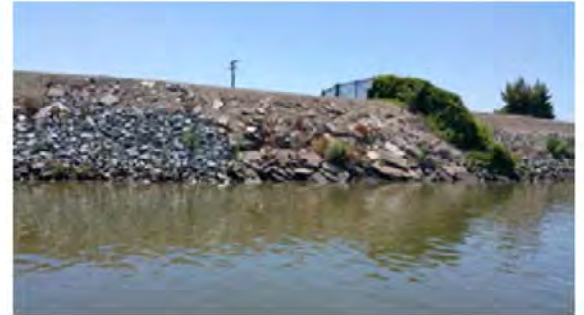
Close view of the erosion.
