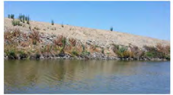
Front view of the erosion.
