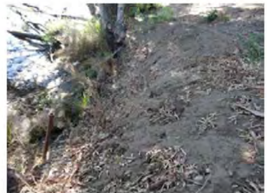
Close view of the erosion at the levee toe.
