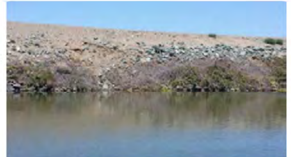
Close view of the erosion.
