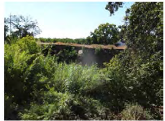
Front view of the erosion. Looking from the right side of the river.
