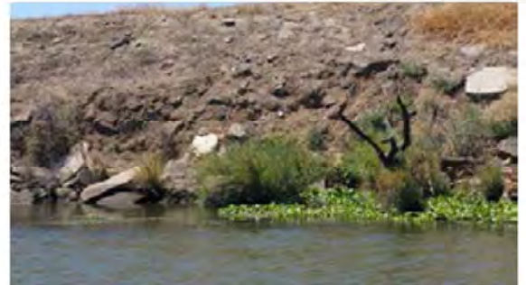
Close view of the pocket erosion.
