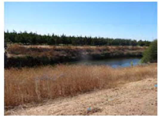
Looking at the erosion from right river bank.
