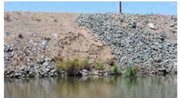
Close view of the erosion.
