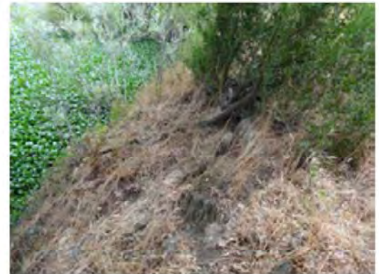
Direct view of the erosion near a tree.
