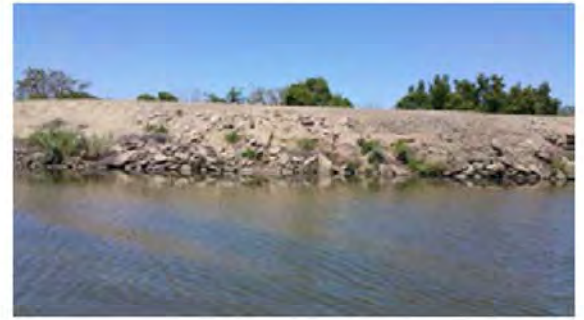
Front view of the erosion site.
