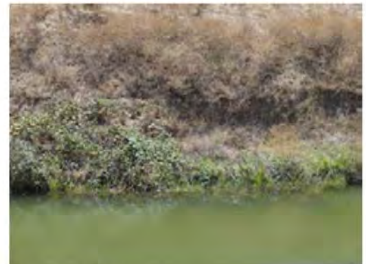
Closer view of the erosion.
