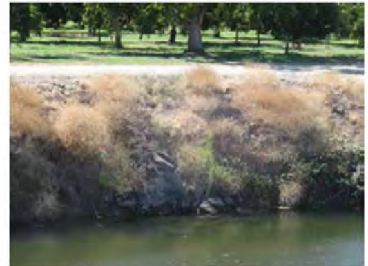
Close view of the erosion. Note the vegetation at the site.
