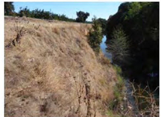
Close view of the erosion site. Small trees grow at the lower slope of the bank.
