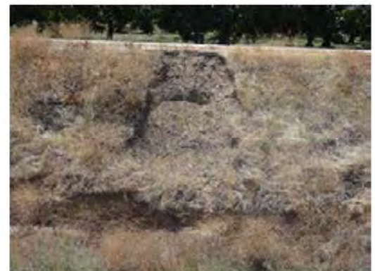
Close view of the erosion.
