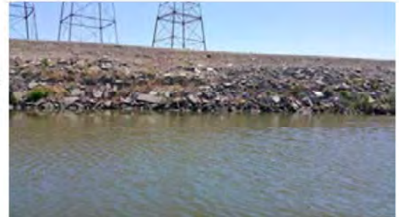
Front view of the erosion.
