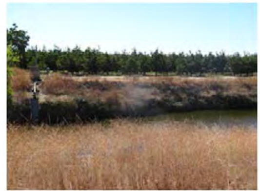
Front view of the erosion
