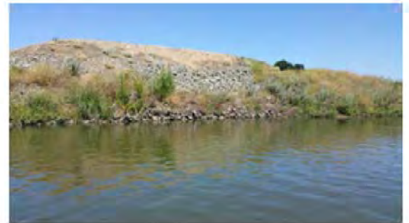
Front view of the erosion.
