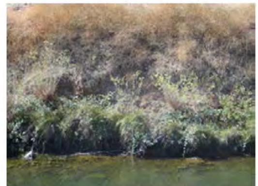
Close view of the erosion.
