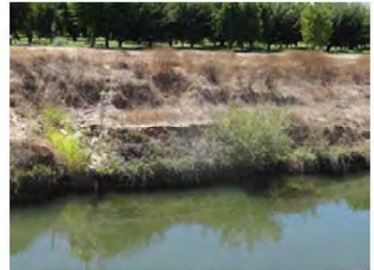
Front view of the erosion at the berm.
