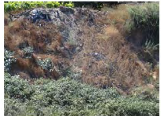
A closer view of the site. Note the pocket erosion immediately next to the repaired site.
