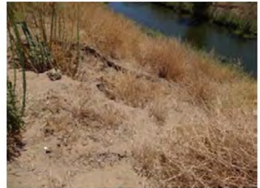
Close view of the erosion.
