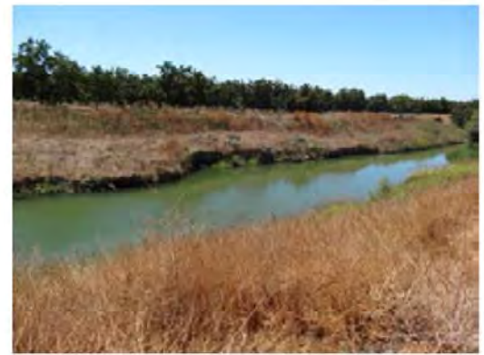
Upstream view of the erosion.
