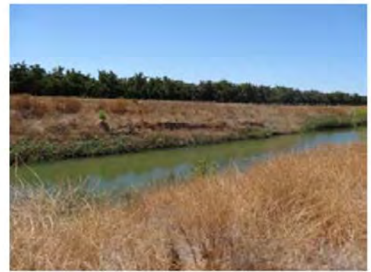
Upstream view of the erosion.
