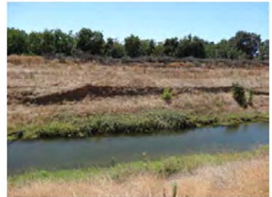
Front view of the erosion.
