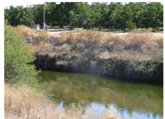
Close view of the erosion.
