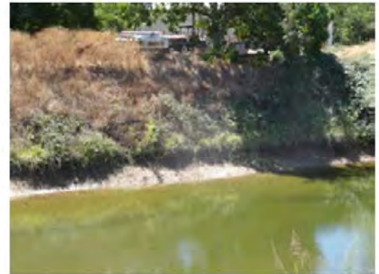
Close view of the erosion.
