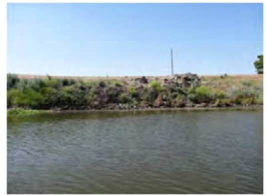
Front view of the erosion.
