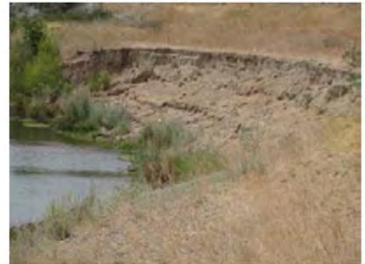
View of the erosion.
