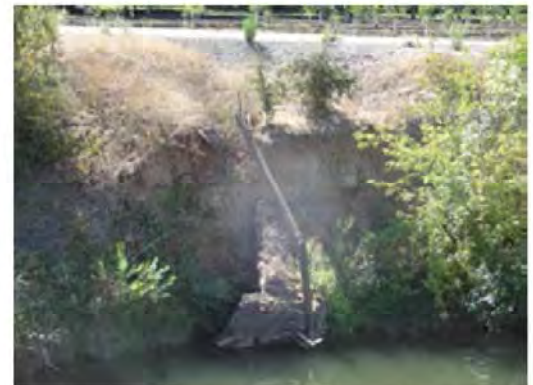
Close view of the erosion. Note the drainage pipe at the site.
