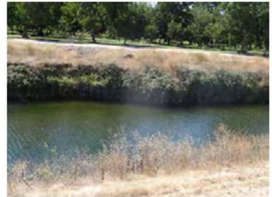
Front view of the erosion. Site is covered with vegetation and trees.
