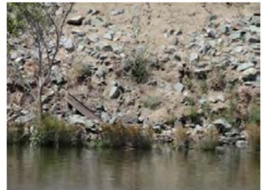
Close view of the erosion.
