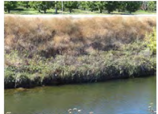
Close view of the erosion.
