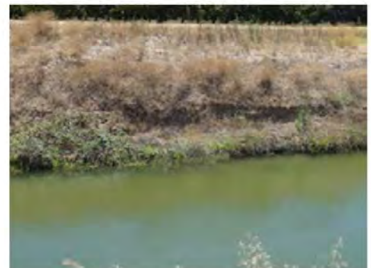
Closer view of the erosion.
