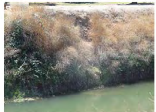
Closer view of the erosion.
