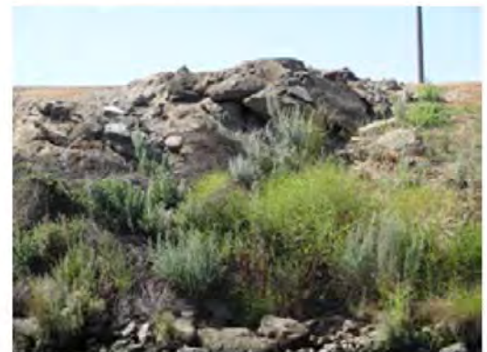
Close view of the site. Note the piled concrete debris.
