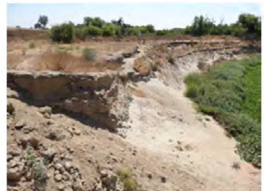
Close view of the erosion.
