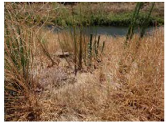
Looking down at the erosion from the levee crest.
