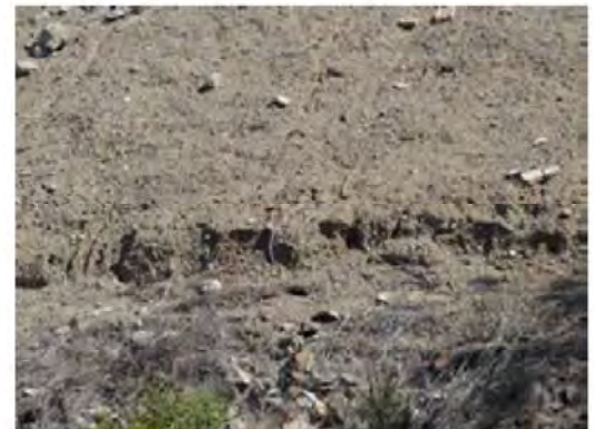
Close view of the erosion.
