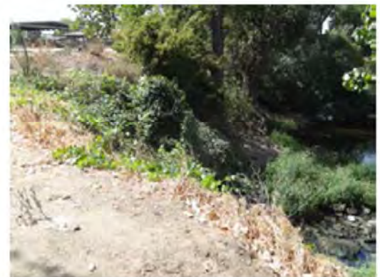
View of the loose material at the bank top.
