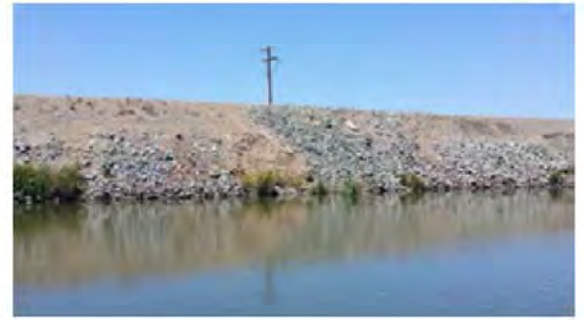
Front view of the erosion.
