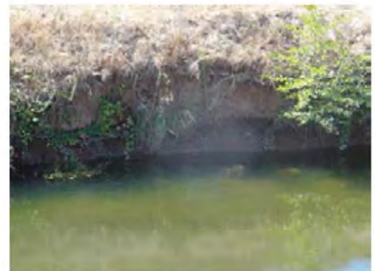
Close view of the erosion.
