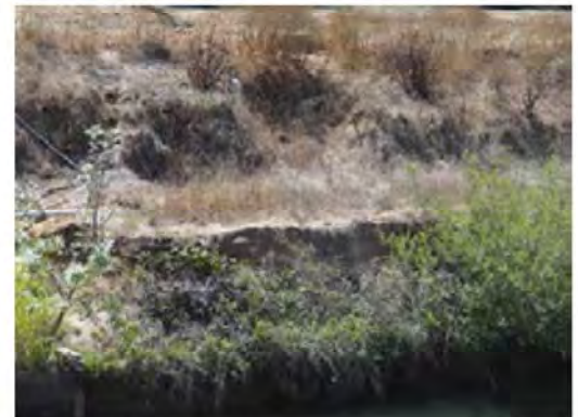
Closer view of the erosion.
